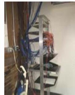
Main Data Rack
