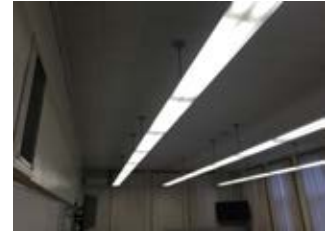
Board Room Lighting
