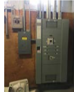
Main Electric Service
