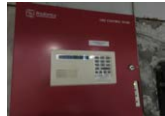
Boiler Monitoring System
