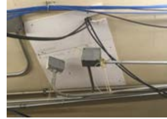
Improperly Supported Boxes
