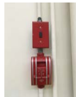
Fire Alarm Devices
