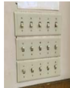
Auditorium Lighting Controls
